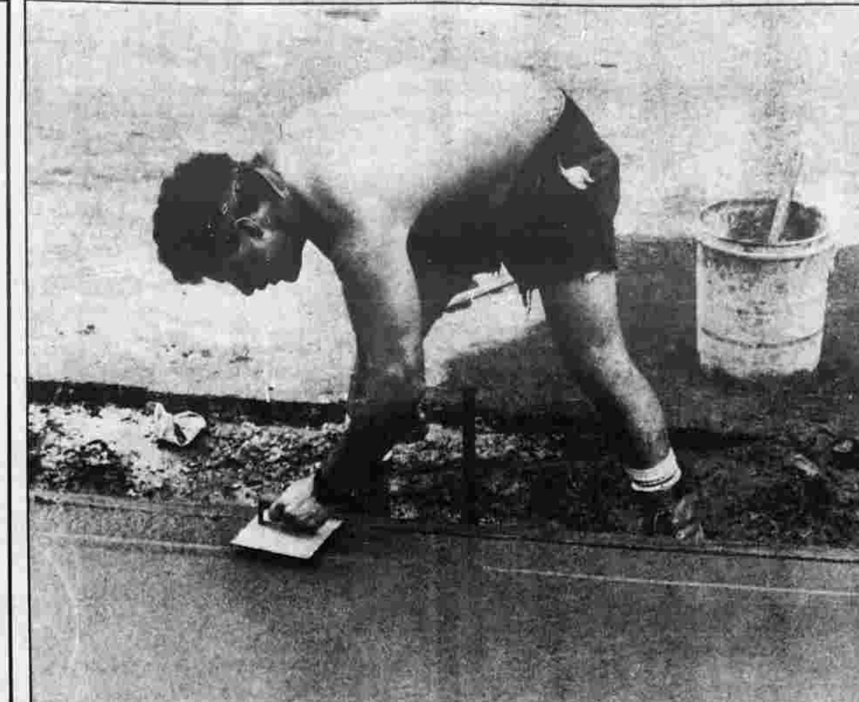
SCULPTING SIDEWALKS — Mark Lapenta of West Hartford, an employee of S. Aleria & Sons, works on the sidewalks on Porter Street Monday. The town is putting in new walks and curbs on the street.
